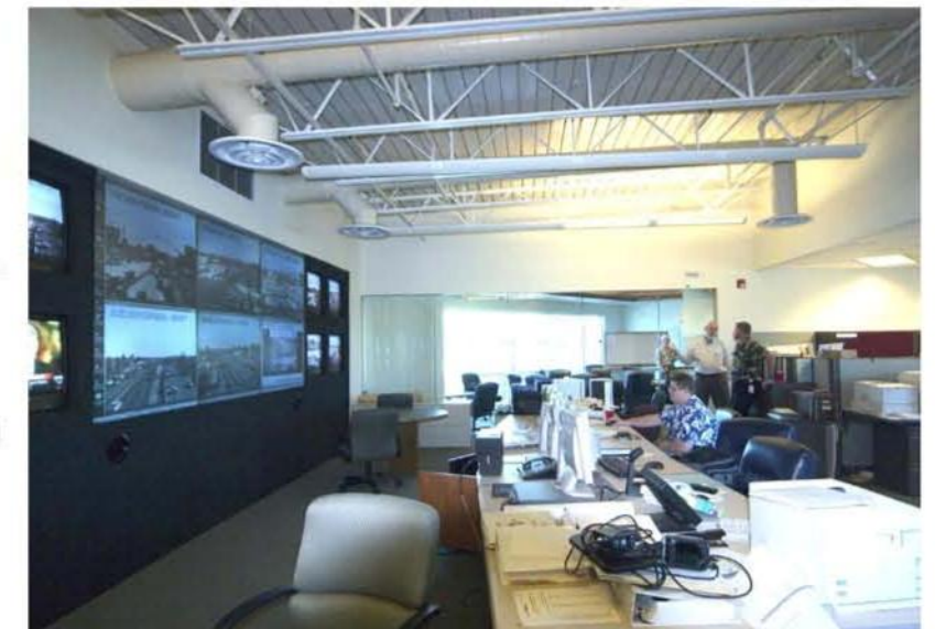
Sacramento County Transportation Management Center
