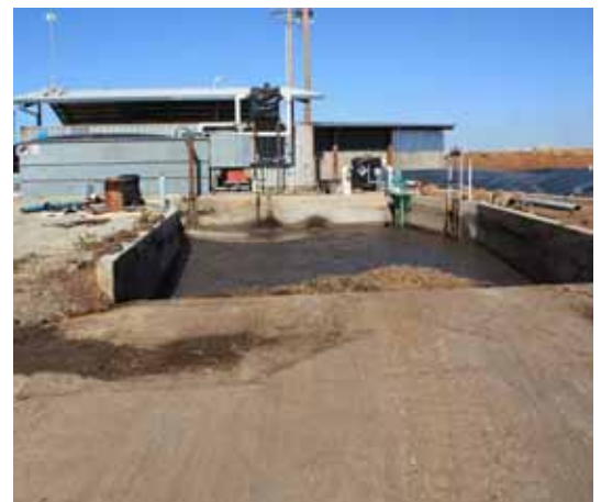
A methane digester (center) uses methane gas from dairy cow waste (right) to power a generator that feeds electricity back into the grid. This innovation provides the Tollenaar Dairy with a stable source of income, a welcome addition given the fluctuating price of milk and other agricultural products. The intake pond (foreground) is designed to handle additional waste, such as food scraps, for the digester.
