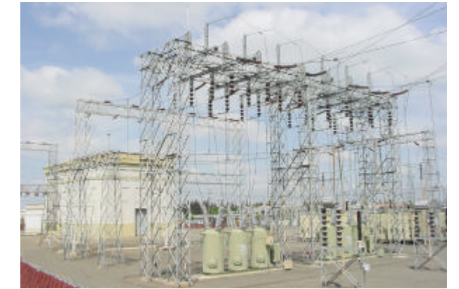
2 - Electrical substation @ Power Inn & Folsom
